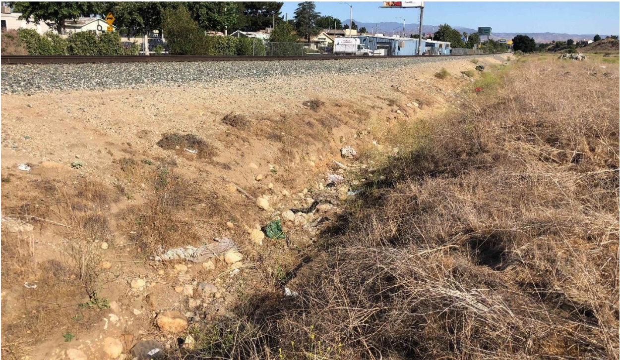
Photograph 8. View of western unnamed drainage feature running parallel to the railroad tracks, facing north. June 10, 2021.
